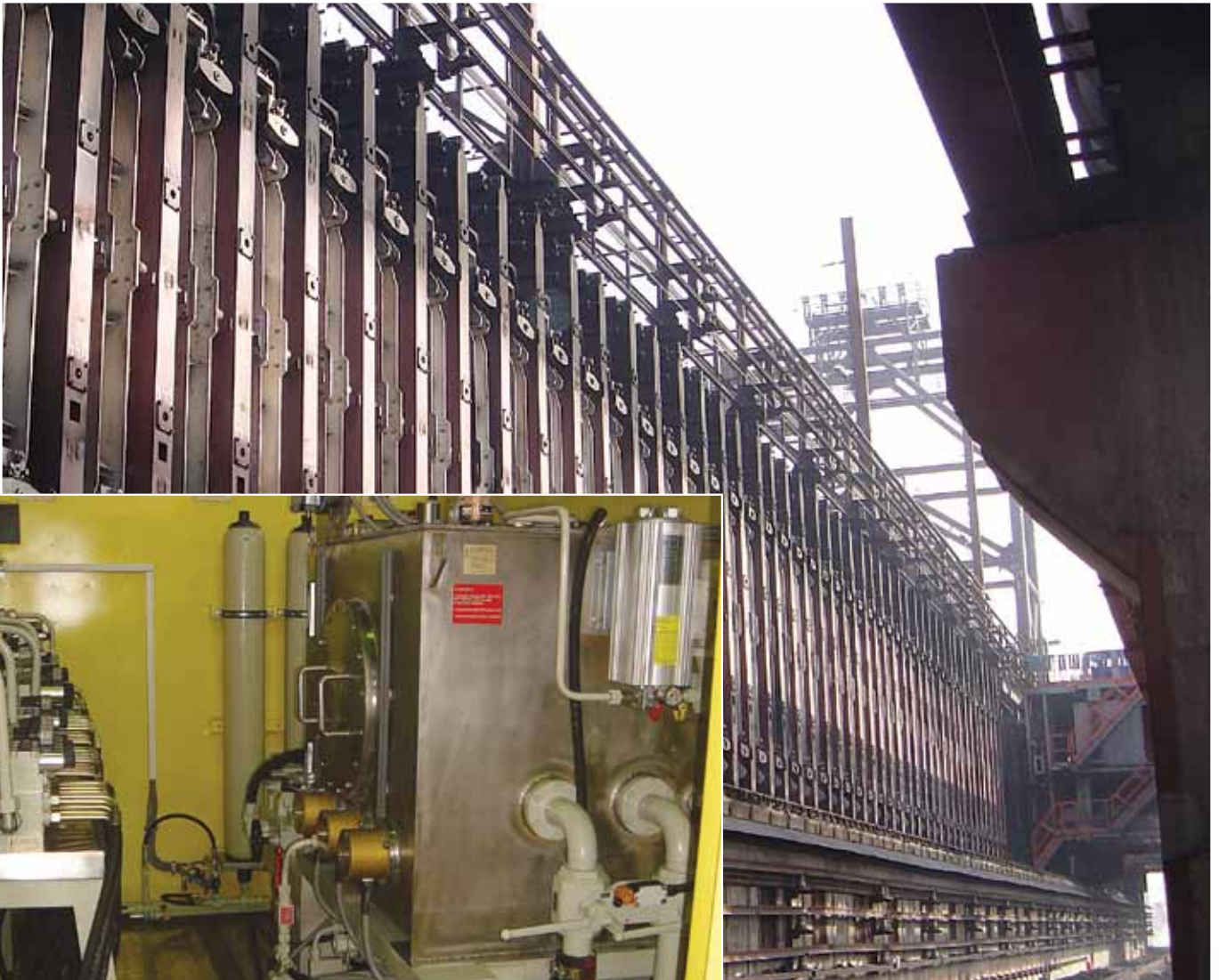
Hydraulic equipment cabin
